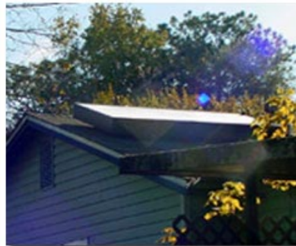
Gainesville – Ms. Robinson’s solar electric panels mounted to her roof use the sun’s energy to heat the water in her home.
